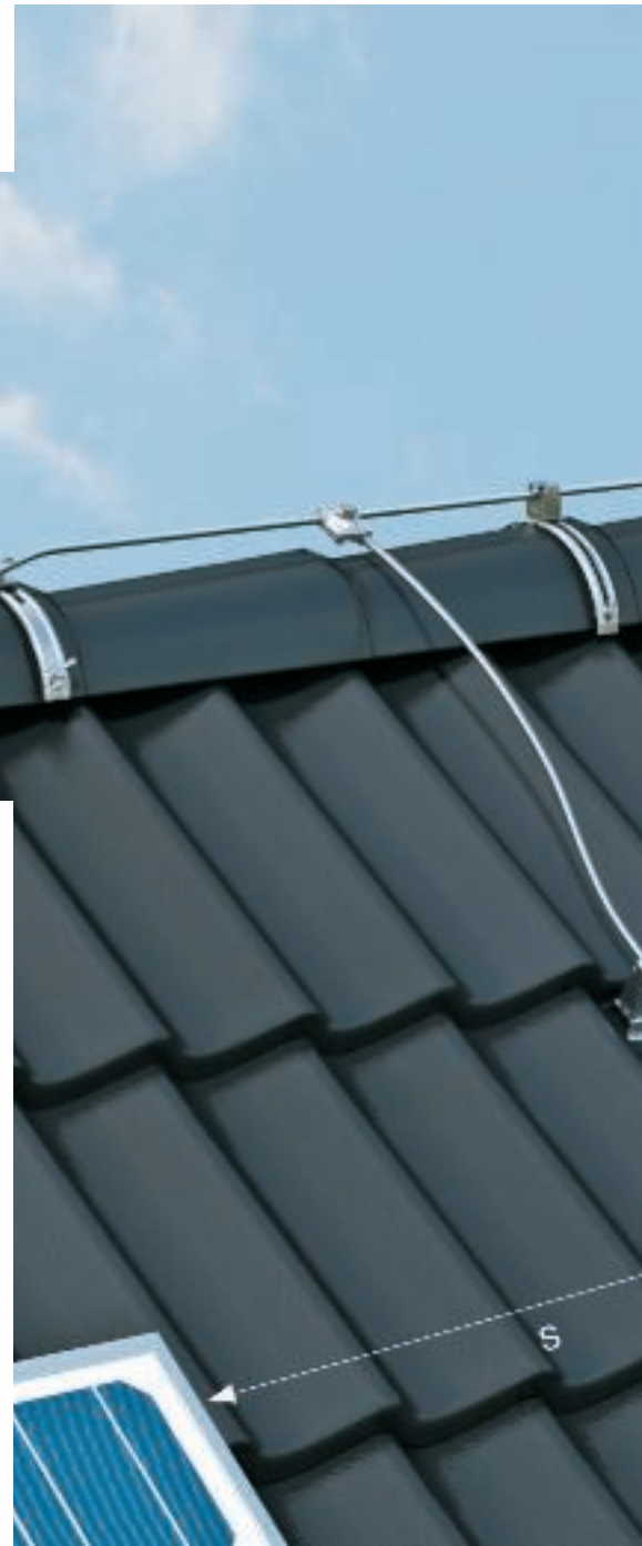
External lightning protection with a PV system installed on a pitched roof
